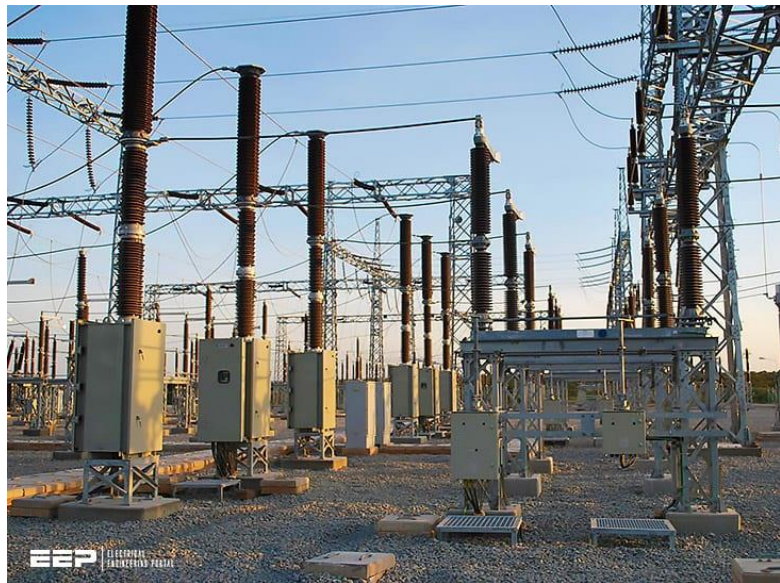
A power substation, much like the ones targeted by TLF. https://electrical-engineering-portal.com/download-center/books-and-guides/power-substations/220kv-substation
